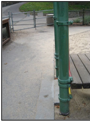
Inadequate fall zone
